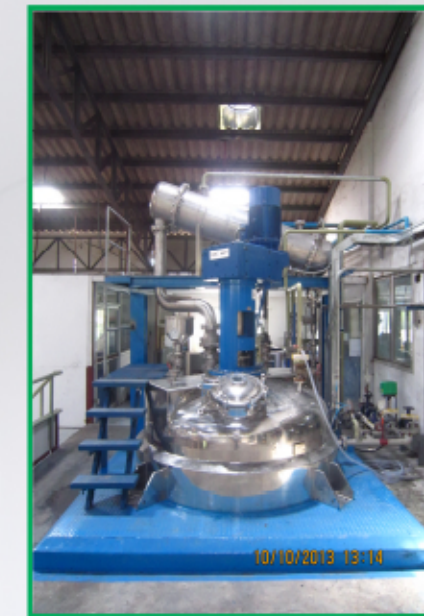
GLUE MIXING TANK 6,000L
