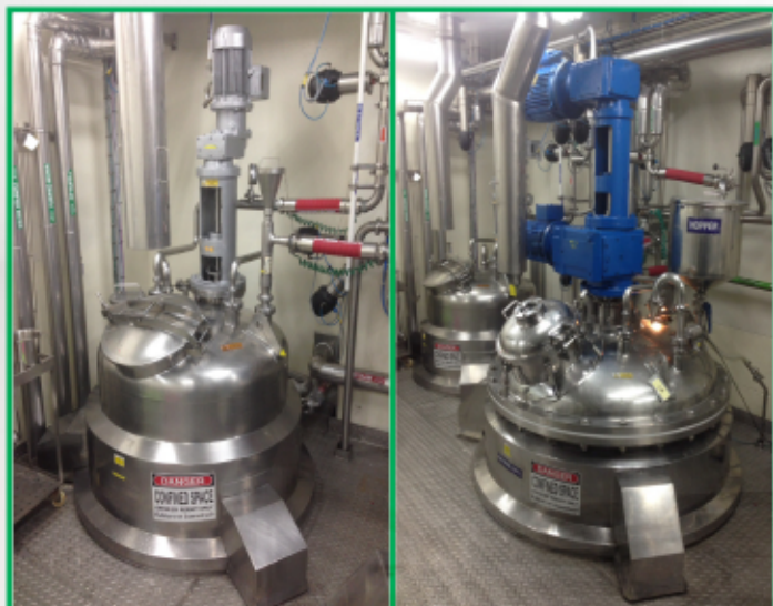
MIXING TANK 2,500L and PREMIX 1,200L
