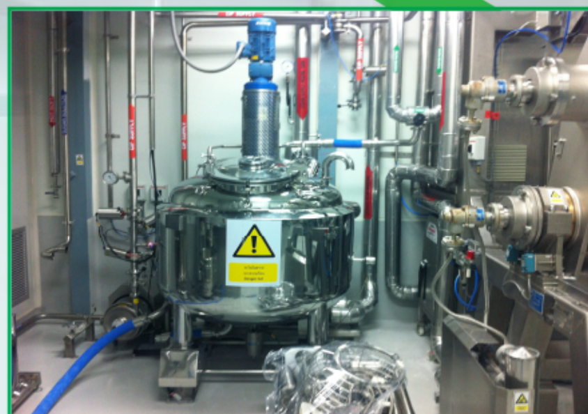
MIXING TANK 1,000L
